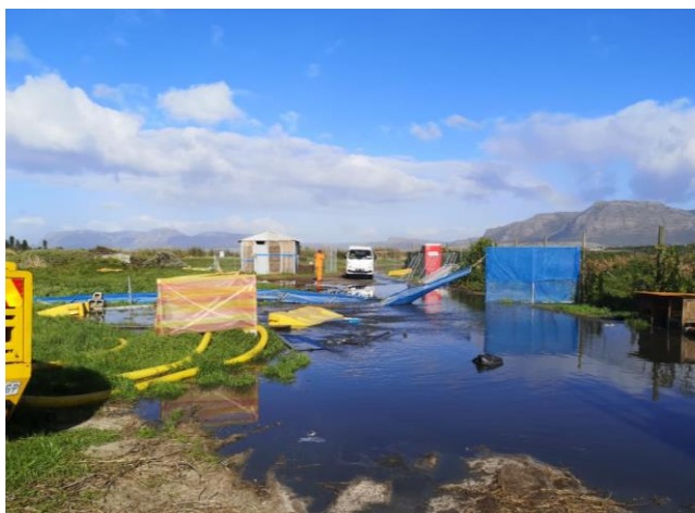
Photo 5.5.1 Attending to a major sewage spill at the Cape Flats WWTW in July 2021, when raw effluent entered Zeekoevlei – a Ramsar wetland
